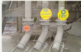
Picture (3): Three pipes to pump the cements up to the silo
